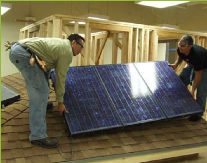
Students installing a solar panel on the roofing display in the solar lab at East Los Angeles Skills Center.
